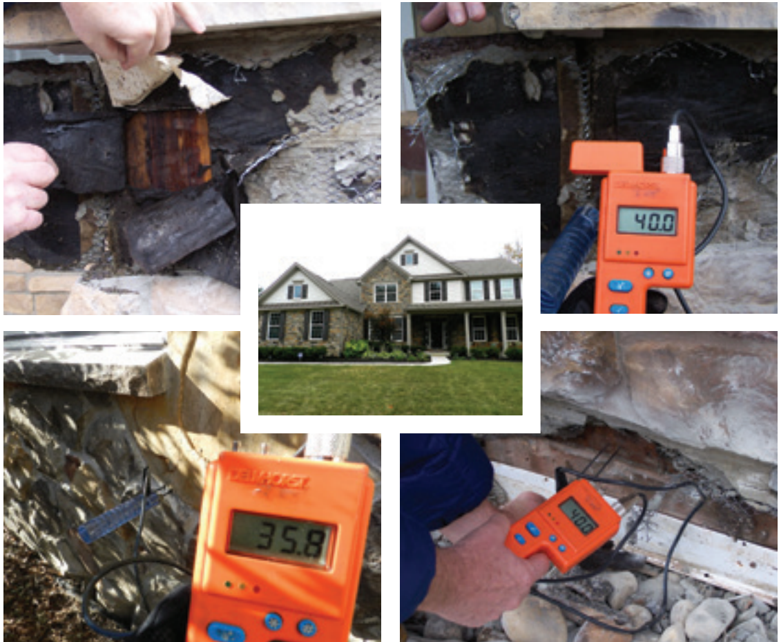
Center: Typical stone veneer; clockwise from upper left: moisture damage behind veneer; moisture probe after removal of veneer; moisture probe at veneer mortar; moisture probe and damage at grade (Photos courtesy of Cliff Kapson)
